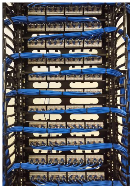
Figure 5.2 – Cable termination at terminating hardware (Backside View).
