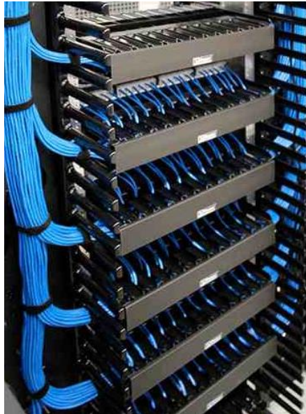
Figure 6.4 – Routing patch cord from cable organizer.
