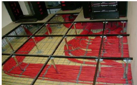
Figure 6.8 – Cable trays deviate (respecting minimum bend radius).
