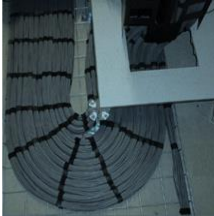
Figure 6.7 – Remainder cable (under rack).
