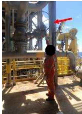
Figure 15. Valve installed above the operator's range.
