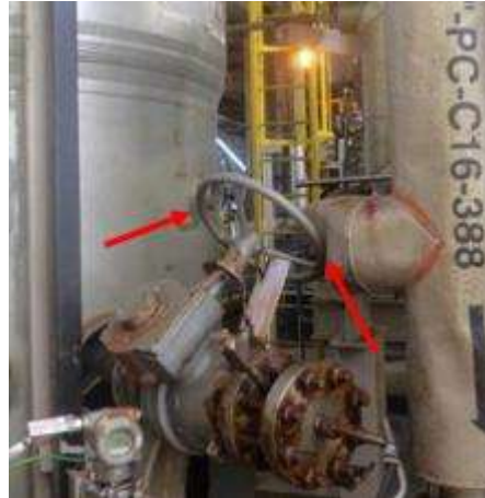
Figure 6. Lack of space around handwheel and inadequate valve position does not allow operator access.
