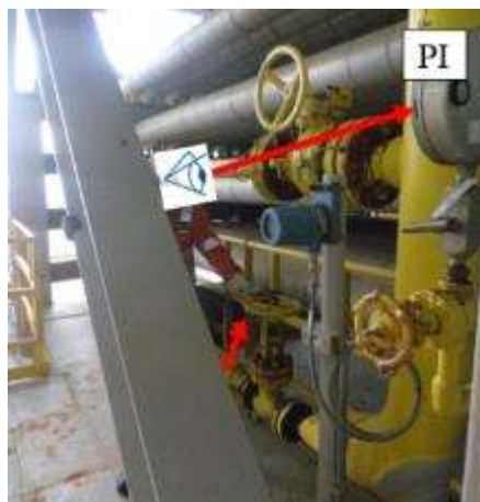
Figure 7. Module support beams restrict access to valves and location of the IP indicator concerning the valve.
