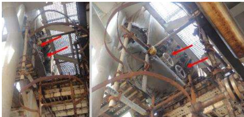
Figure 25. Improper position of category 1 valves.
