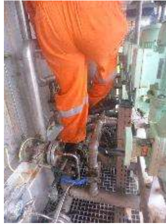
Figure 4. Valves installed in a place where access requires permanence on pipes and equipment.
