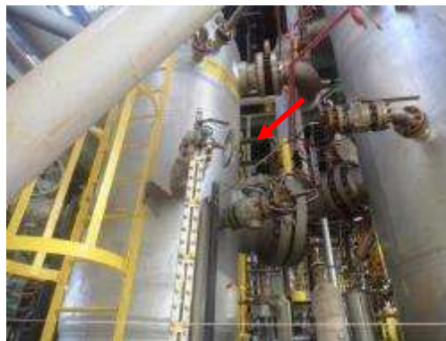
Figure 23. Valves installed on the opposite side of ladder, making it difficult to access.
