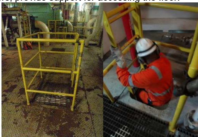
Figure 19. Vertical ladder with support for accessing engine room’s last level.
