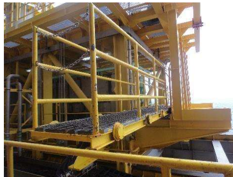
Figure 17. Retractable walkway to access the trolley
