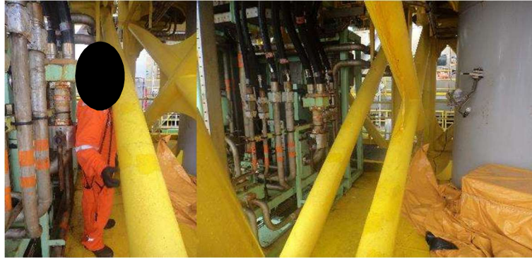
Figure 18. Obstructed access to the electrical panels of auxiliary hoist
