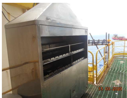
Figure 12. Barbecue adjacent to the messroom, coverage and side protection are needed.
