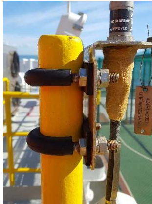
Figure 1 – Example of cable fixing
