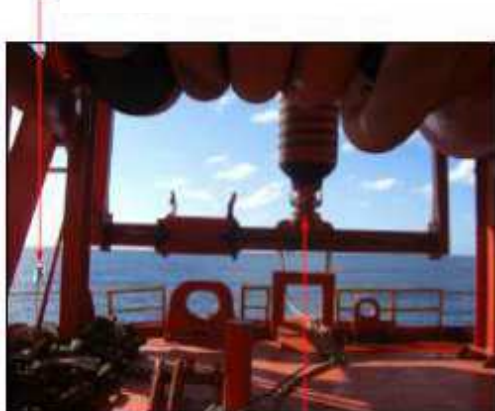
CENTER HOSE (AFT)
