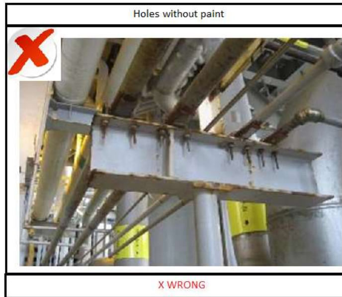
Figure 8 – Hole for bolts drilled with no precaution for not damaging the paint and with no preservation during assemble
