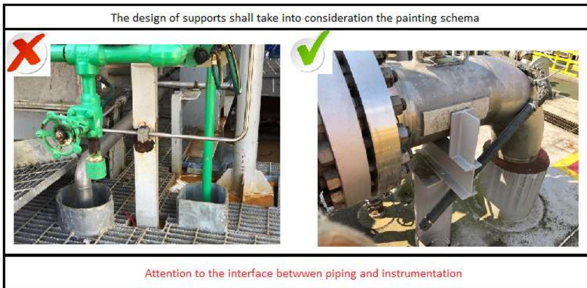
Figure 15 – Carefully with piping and instrumentation interface
