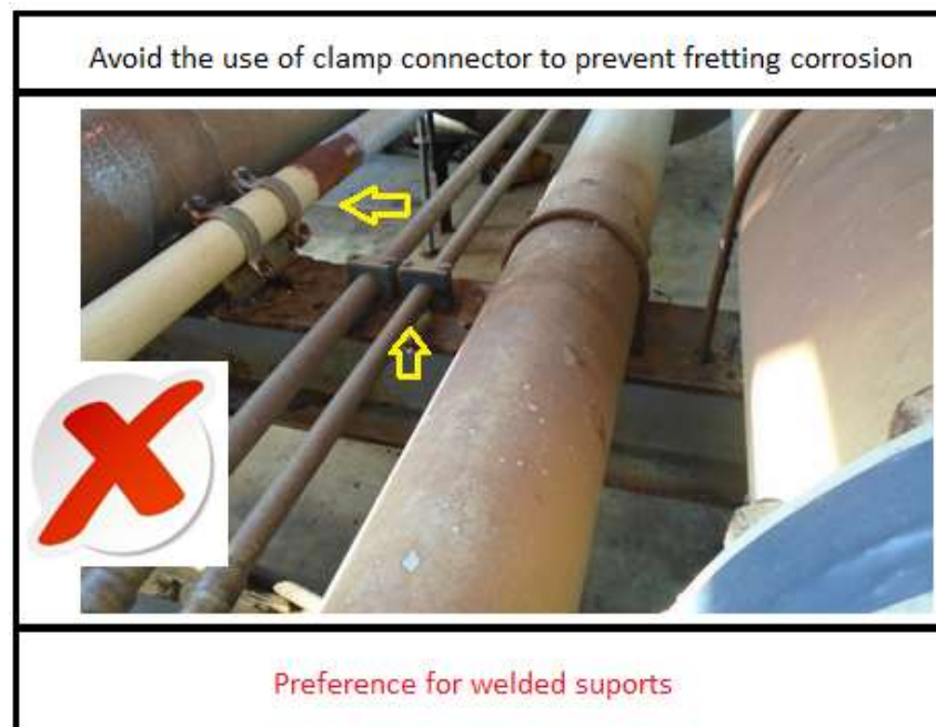
Figure 9 – The use of clamp supports shall be avoided
